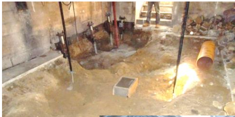
Residential Basement Cleanup
